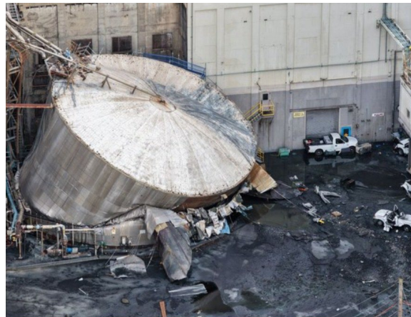
The collapsed white liquor tank at the Longview mill.
